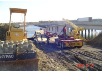
Beams were loaded onto barges and then erected by a barge-mounted crane.
